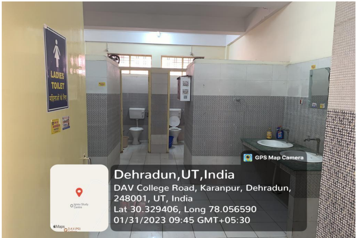
Ladies Toilet with Napkin Dispenser and Incinerator
